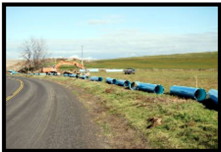
Piping Eastside delivery system
