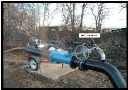
New metered pumping station
